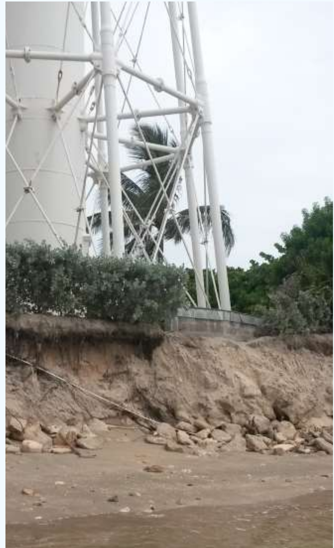
HLPS Shore Erosion, Sept. 28, 2015
